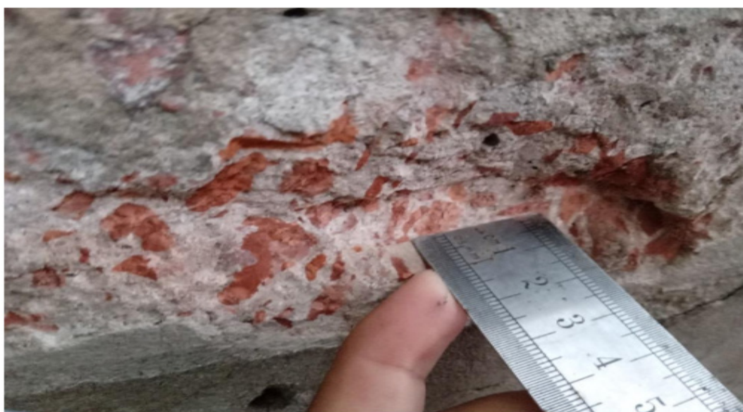
Figure 1: Physical measurement of fire-induced crack depth (approximately 8 mm) at a column face using a feeler/ruler technique.
