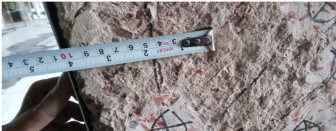
Figure 2: Tape measurement of a fire-induced column crack (approximately 105 mm) prior to correlation with the corresponding UPV-estimated crack depth
