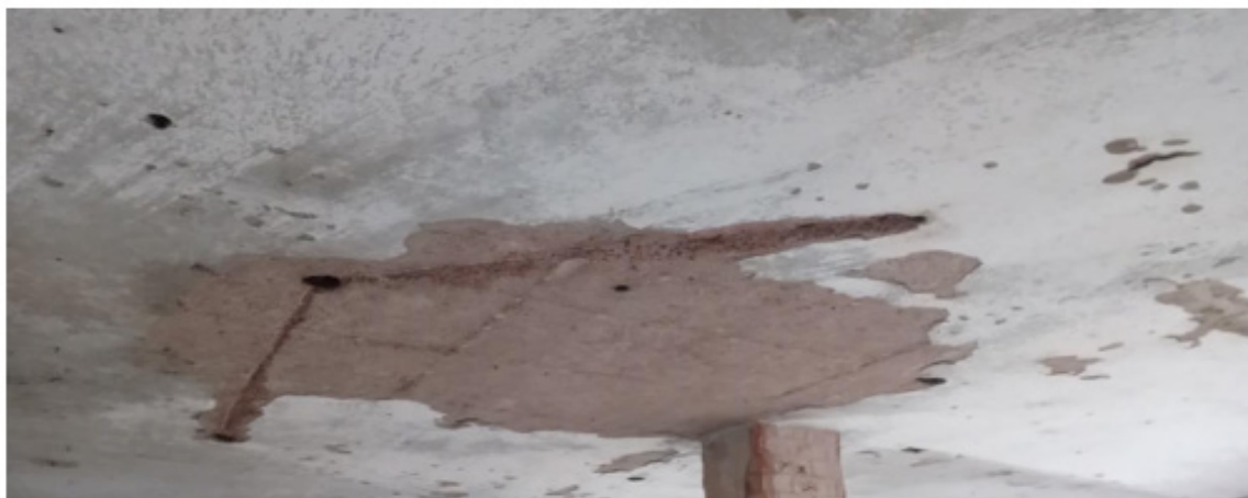
Figure 3: Spalling of soffit plaster on the third-floor flat-plate slab, typical of the surface-only distress observed across the slab away from the toilet zone.
