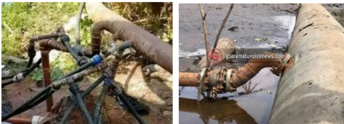
Figure 5: Siphoning Crude Oil from a Pipeline (Princely, 2022).
