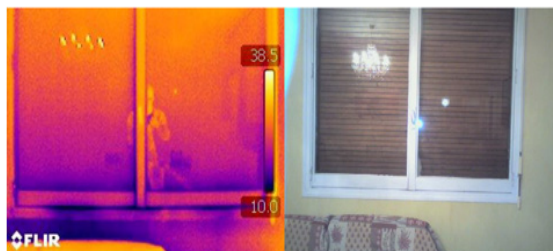
Figure 24: Lack of airtightness on joinery
