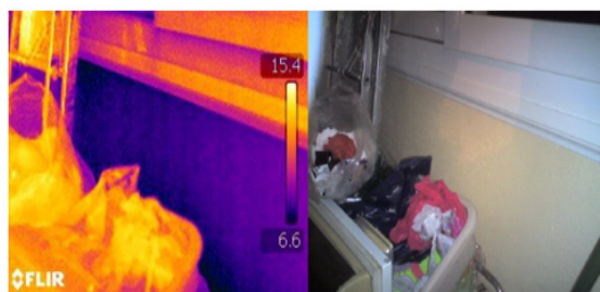
Figure 25: Heat loss from uninsulated walls
